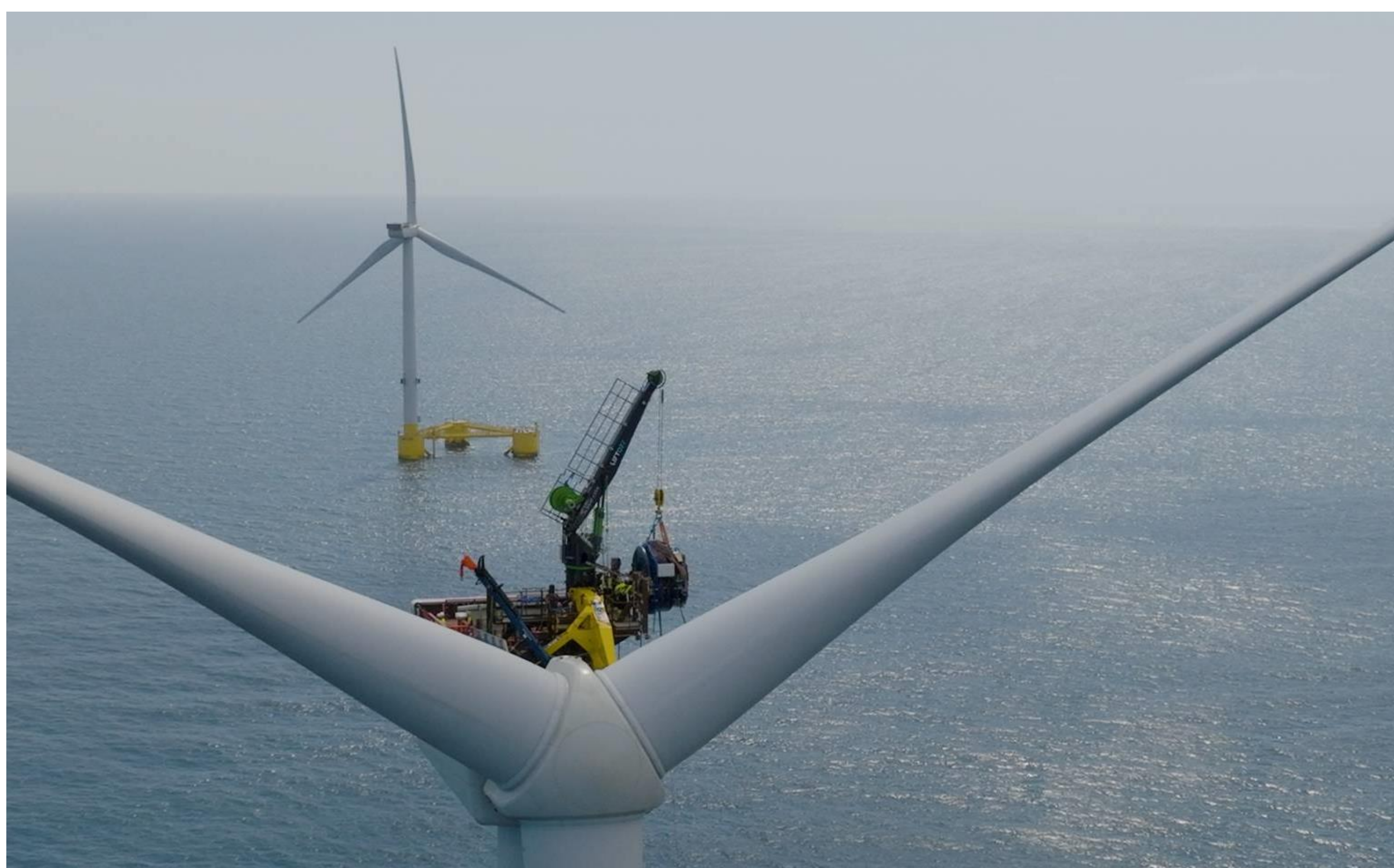
Self-erecting crane from LiftOff at Kincardine Offshore Wind Farm in 2024 (Credits: Cobra).
