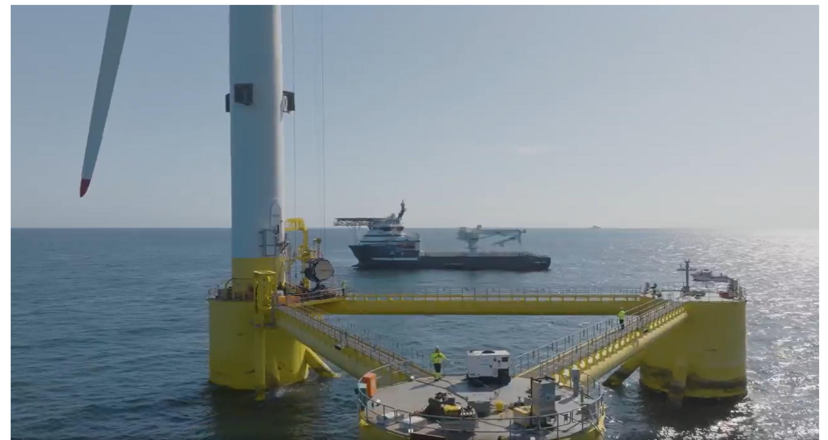
In-situ WTG major component replacement at Kincardine Offshore Wind Farm (Credits: Cobra).
