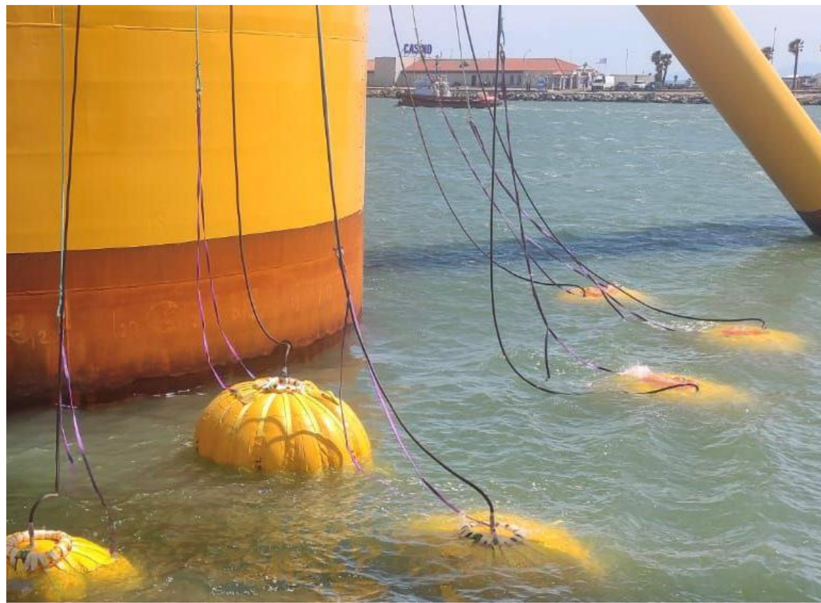
Lift bags at EFGL (Image: Rana Subsea)
